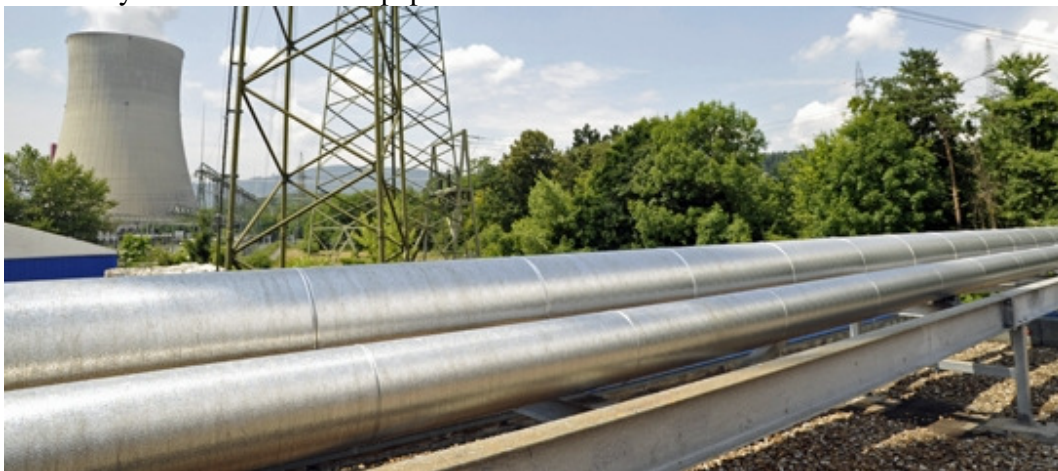
Figure 3-7: Pipeline from Gösigen NPP to Aare paper mill (Kernkraftwerk Gösigen-Däniken AG 2011).
