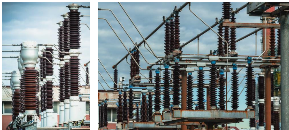
Figure 2: High Voltage switch and High Voltage disconnector at the primary substation Raffinerie
