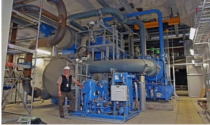
Figure 9-9 90 MW thermal, heat pump feeding Helsinki District Heating 110
