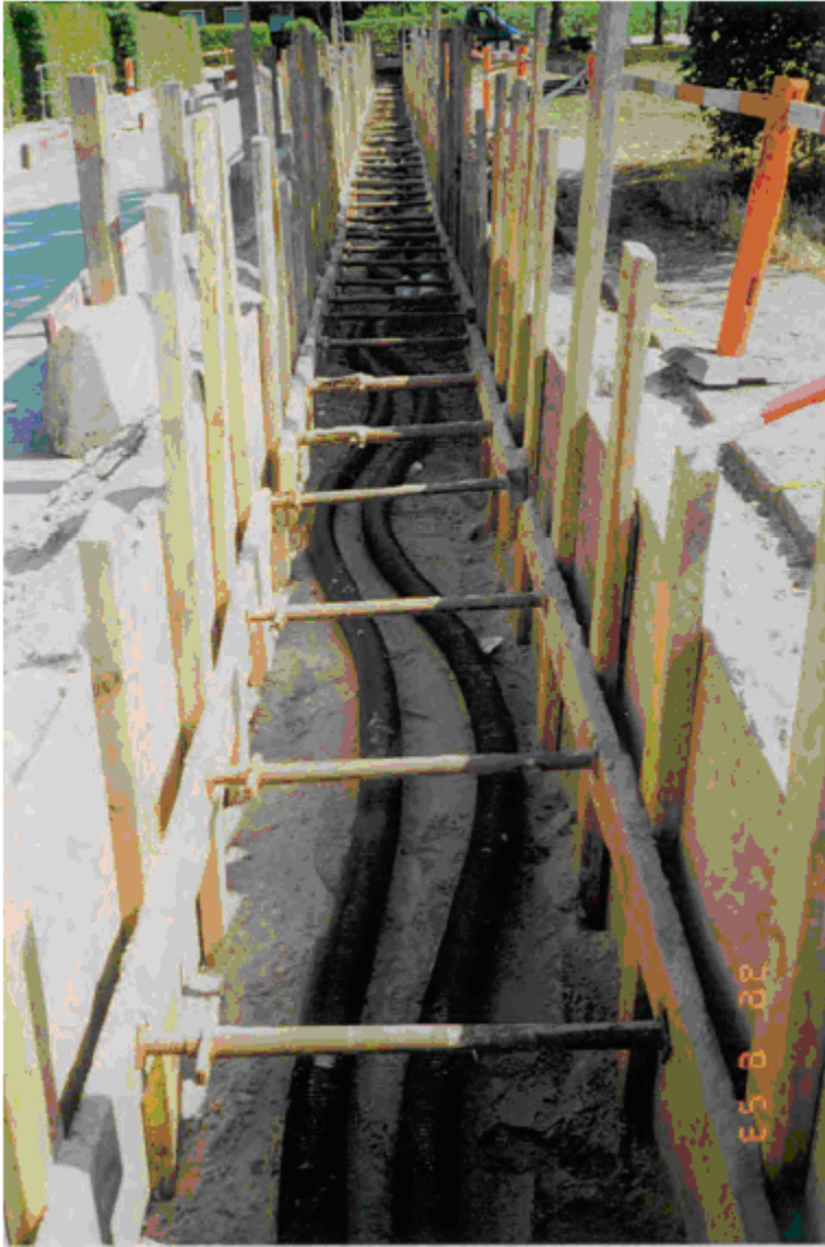
Figure 13-1 Modern plastic low temperature DH pipe. Laying the pipes in a curve means thermal expansion joints are unnecessary 161
