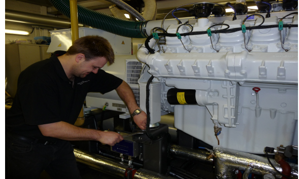
Figure 20-1 Approx 500 kWe gas engine chp unit
