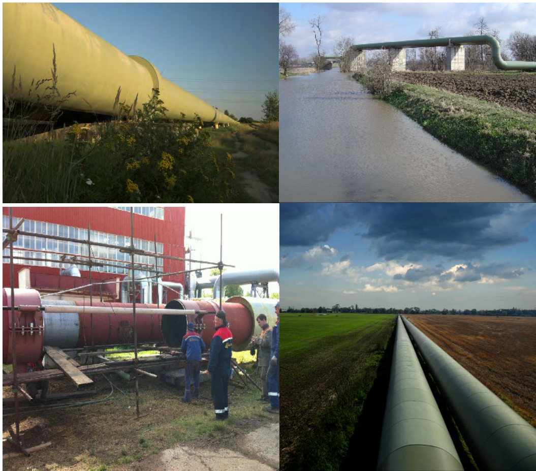
Figure 12-4 Melnik-Prague heat main (2 x DN 1200). The distance is almost 40 km to the Prague city gate and 64 km to the opposite city gate. It was started in 1996. 156
