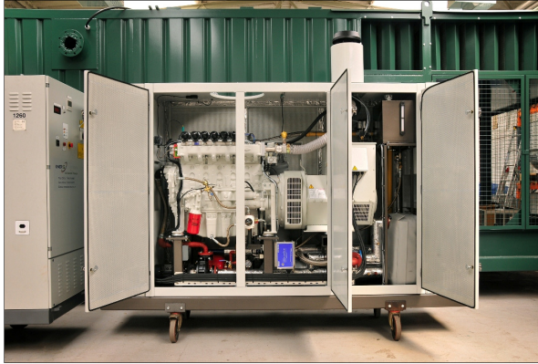
Figure 20-2 Approx 150 kWe gas engine chp unit
