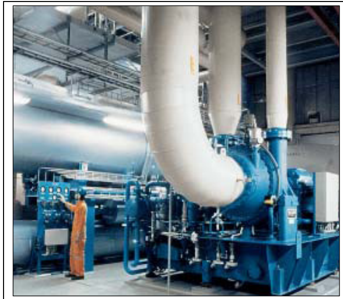
Figure 9-10 180 MW thermal, heat pump feeding Värtan Ropsten District heating plant part of Stockholm District Heating. 111
