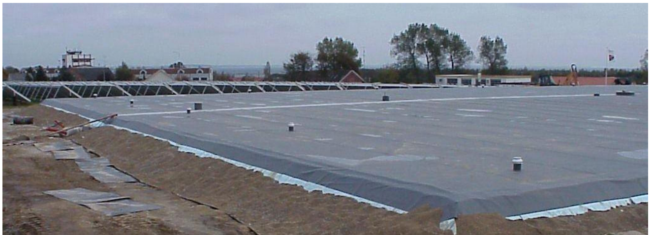
Figure 10-4 10.000 m2 pit storage in Marstal District heating Denmark 127
