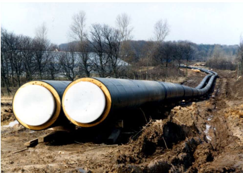
Figure 12-1 Bulk transmission pipes being installed – notice thinness of insulation on large pipes. 147
