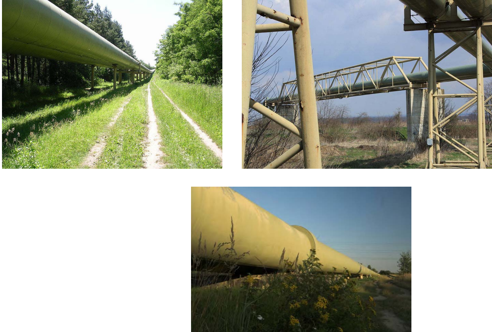
Figure 3.5: 60 km, 2 x DN 1200 pipe delivering 200 MW from Melnik to Prague DH 27
